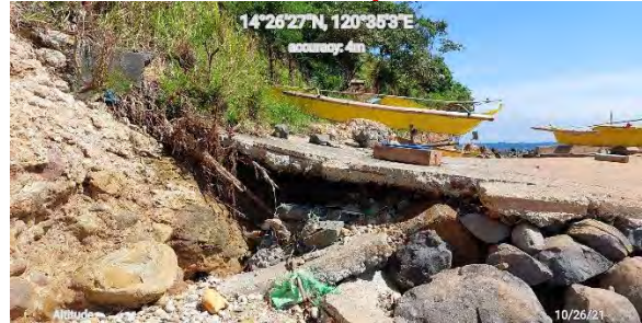
Collapse of the community boat landing areas due to high waves during the onset of typhoons
